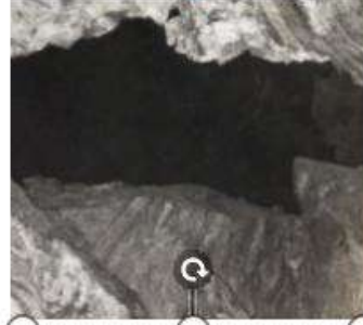
Seriously fractured rock
